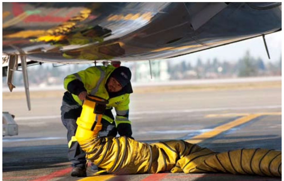
Providing heating and cooling to our aircraft parked at the gates is now achieved with ground power rather than the aircraft's auxiliary power unit. This saves an estimated 2.7 million gallons of fuel per year. Photo: Don Wilson, Port of Seattle.
